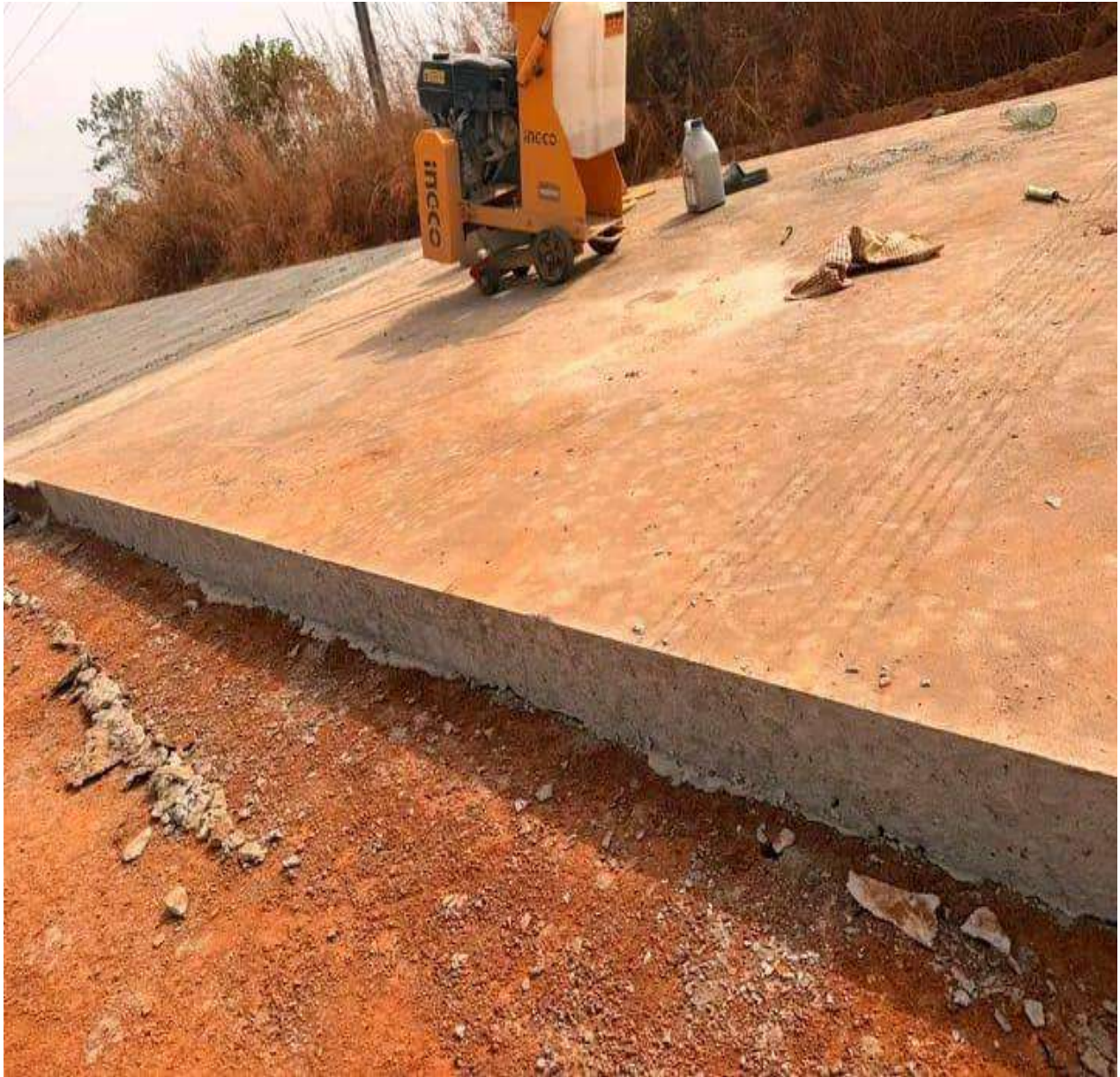
Fig 5.1 Construction of 17.1km Isu-orieagu -obeagu, ezzagu Road (15cm Rigid pavement thickness and Hydraulic structures) Onicha LGA
