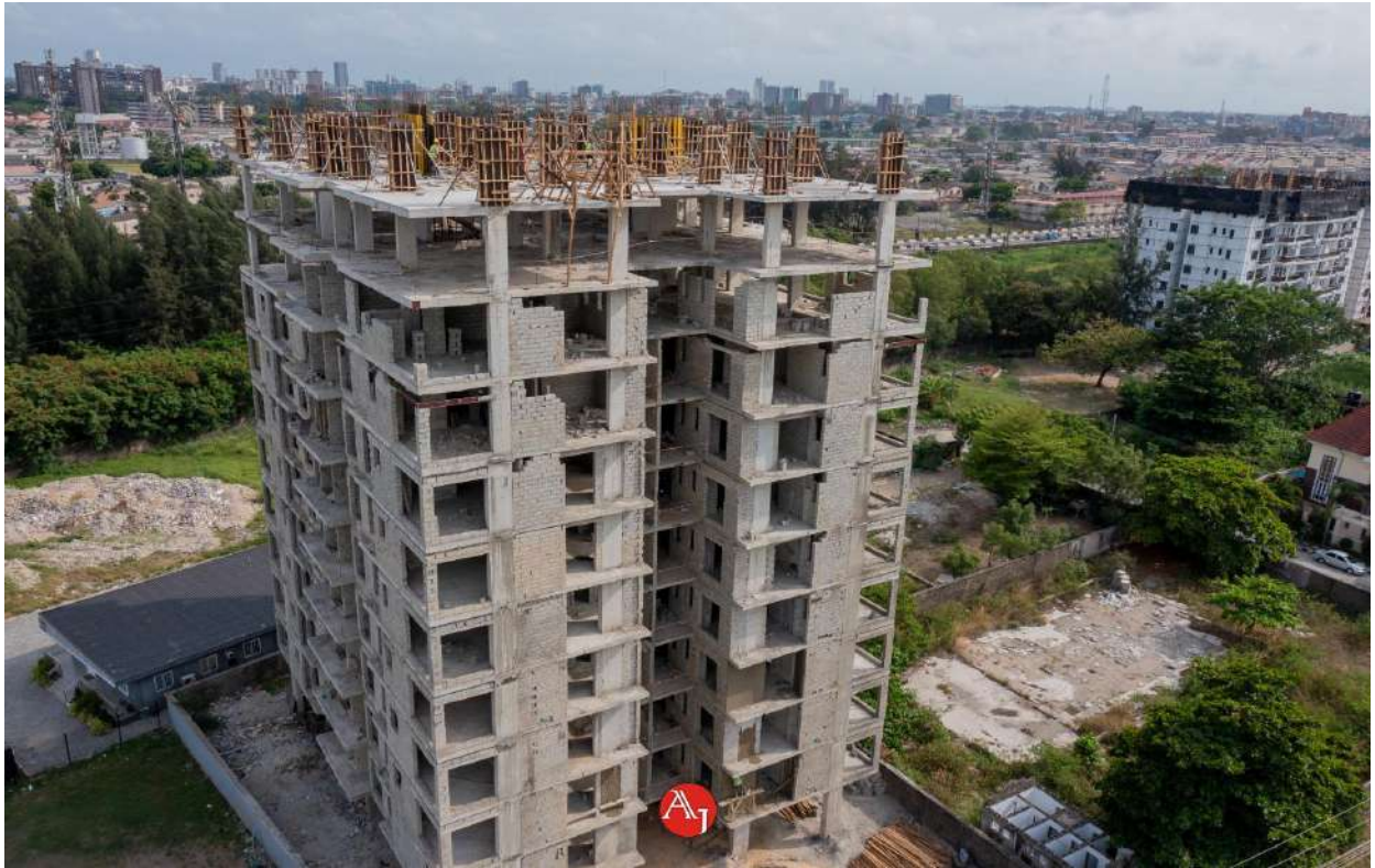
Fig. 6.1 Construction of a Residential Development at Osborne, Osborne Foreshore water Estate, Ikoyi
