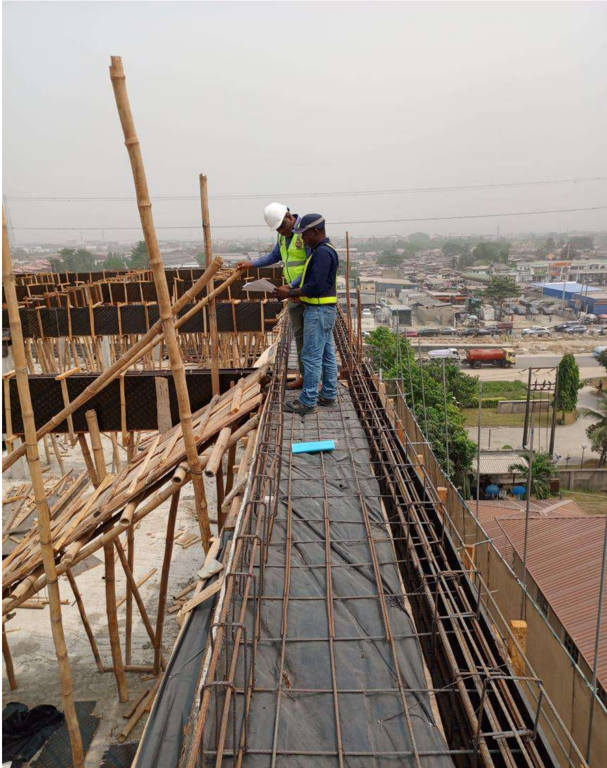
Fig. 5 SWISSTUNA office complex, at Ikota, Eti-Osa LGA. Lagos.(Roof beam and Parapet wall Reinforcement laying)
