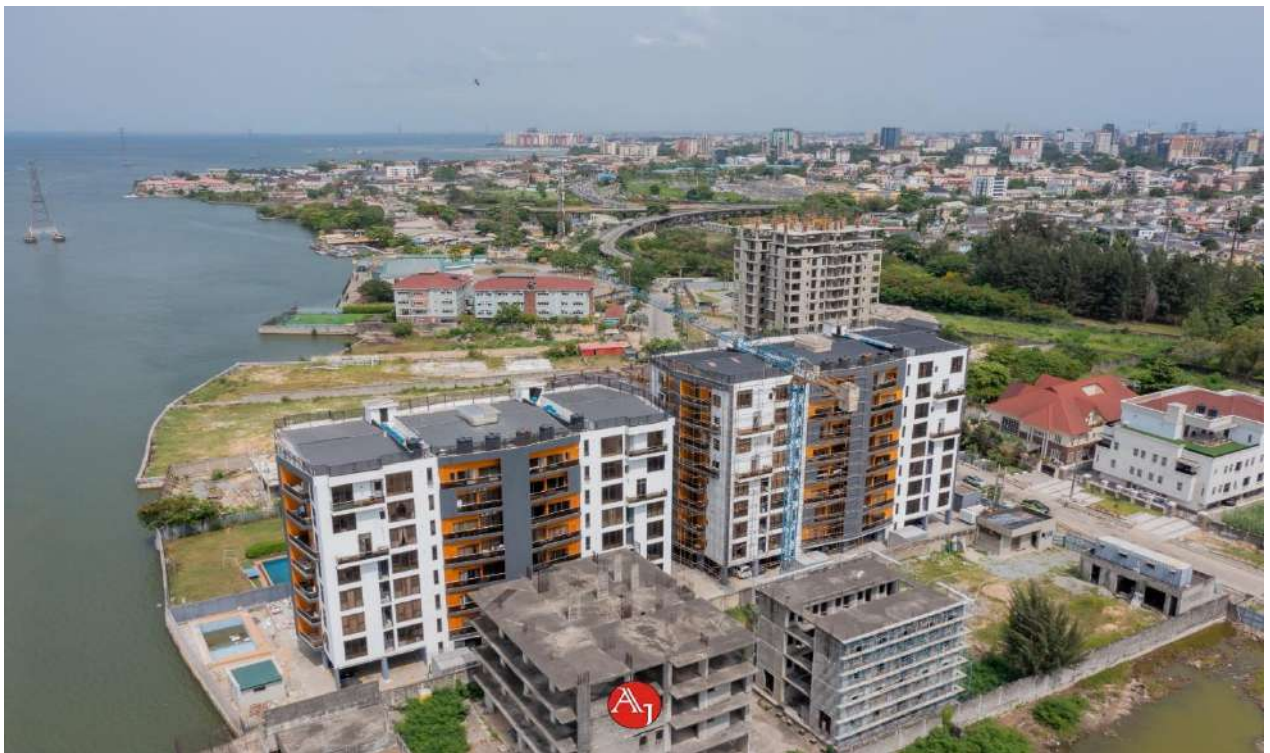
Fig. 6.2 Construction of a Residential Development at Osborne, Osborne Foreshore water Estate, Ikoyi
