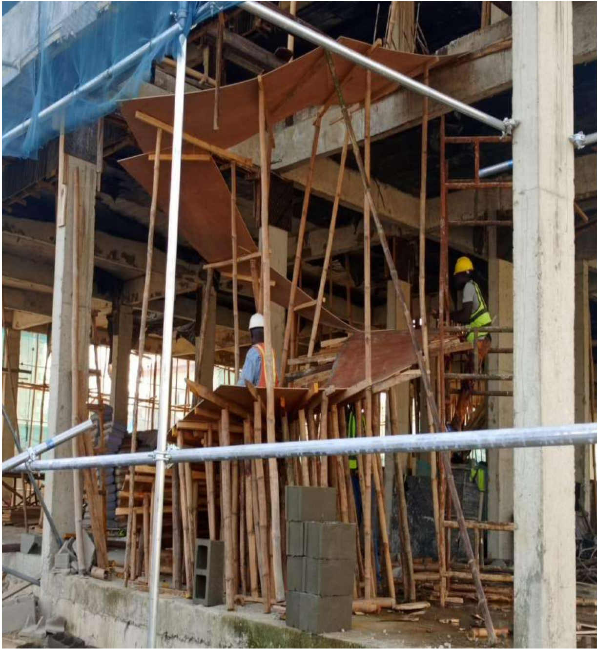
Fig. 7 SWISSTUNA office complex, at Ikota, Eti-Osa LGA. Lagos. (Preparation of Spiral staircase on the ground floor)
