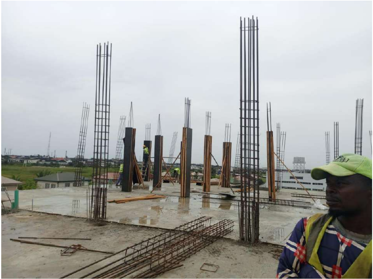
Fig. 8 SWISSTUNA office complex, at Ikota, Eti-Osa LGA. Lagos.(Preparation of columns reinforcement on second floor)
