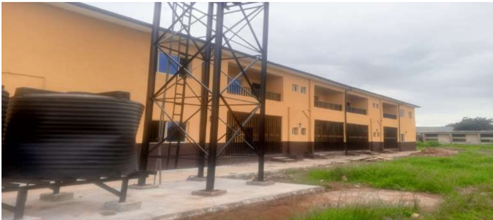
Fig: 01 Renovation of Auditorium building at nwafor orizu college of education nsugbe, Anambra state.
